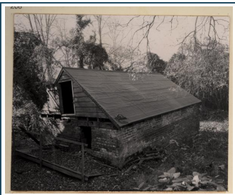
THE STOREHOUSE BEFORE ITS RESTORATION, AS SEEN FROM THE NORTHEAST. AN OLD "WINDOW" OPENING STILL EXISTED IN THE EAST WALL. IT WAS NOT BELIEVED THAT THE PATCHED AREAS IN THE NORTH WALL HAD BEEN WINDOWS, SO THAT NO BASEMENT WINDOWS WERE PLACED IN THIS WALL WHEN THE BUILDING WAS RESTORED.
