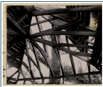
VIEW OF ROOF FRAMING FROM WITHIN THE OFFICE, MADE DURING THE RESTORATION OF THE BUILDING IN THE LATE 1930'S. THE PLASTER CEILING HUNG ON THIS FRAMEWORK HAD THE APPEARANCE OF A SHALLOW GROIN VAULT.
